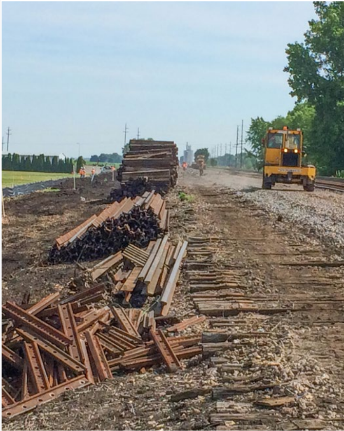
RailWorks employees remove rail at Union Pacific's Athol siding in Lincoln, IL, as part of upgrades to the high-speed rail corridor between Chicago and St. Louis. RailWorks is removing and replacing 2 miles of track, timber ties and two industry spurs in Lincoln to make way for new track consisting of 130-lb. rail and concrete ties.
