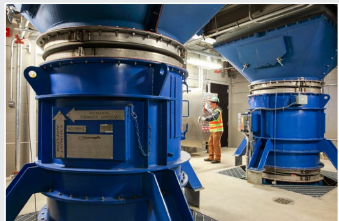
Foreman Patrick Ritter works in the Capitol Hill Station fan room to check the wiring of the control panel for fans and dampers. The large blue fans are part of the Emergency Ventilation System and control exhaust air flow in the train tunnel.
