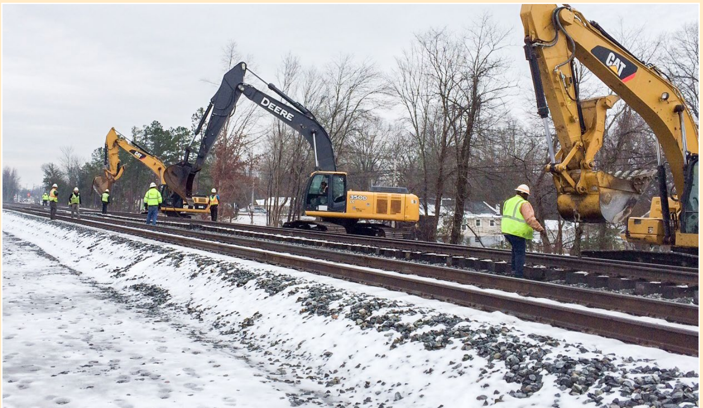
As part of the construction of a second NS mainline between Reid and Kannapolis, NC, RailWorks crews positioned 200-foot track panels that comprised a temporary detour track.
