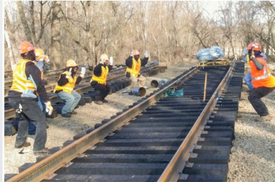
A group of newly hired Central Region employees, led by Laborer Chris Jarmon, stretch prior to constructing track in April near a Cargill grain elevator in Savage, MN.
