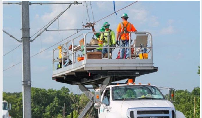
During a cutover in July, L.K. Comstock workers completed the interface of the newly installed overhead catenary system on the Dallas Area Rapid Transit agency's new Blue Line extension with the existing Blue Line.
