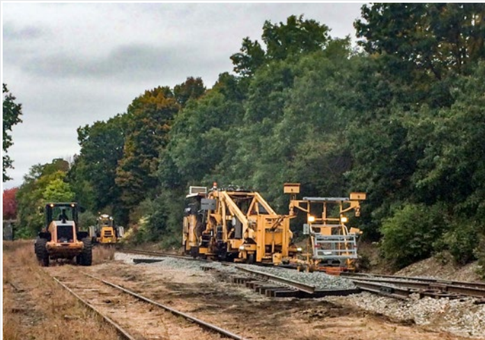
This turnout in Willimantic, CT, is one of nine that RailWorks is installing on the New England Central Railroad.
