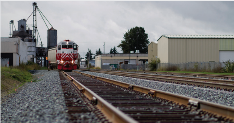
RailWorks Track Systems is wrapping up work to reconstruct the track for Sound Transit's M Street to Lakewood commuter rail project. While work continues on the line, freight trains operate from Thursday evening through Monday morning.
