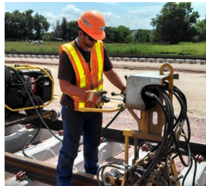
Evan Klein spent much of his summer laying ties at the new oil-loading terminal for Eighty-Eight Oil LLC in Fort Laramie, WY. Evan, an Oregon State University junior majoring in energy systems engineering, said he appreciated his freedom to accomplish a job the way he thought he should while still having people accessible to answer questions.
