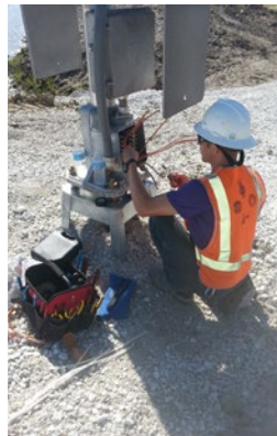
Intern Steven Castello, based out of Jacksonville, FL, worked on projects including SunRail signal maintenance and fiber cable installation on Florida East Coast Railroad. The Michigan Tech senior found value in seeing "how things operate on a large scale and the organization needed even for the smallest things."
