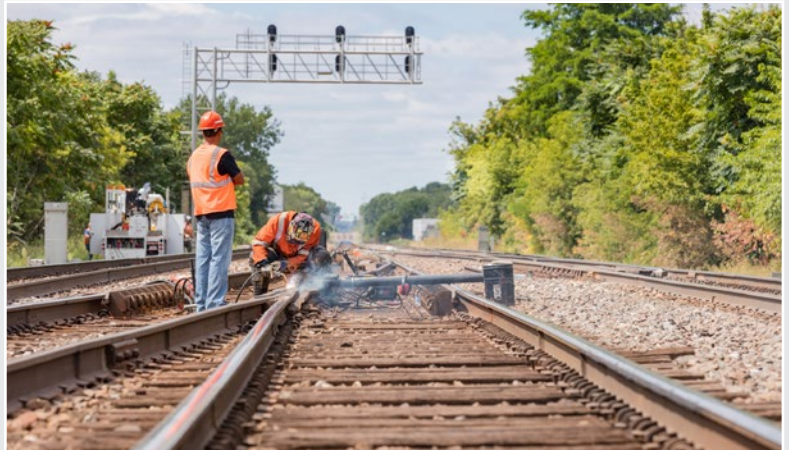
Helper Eric Balsler performs electric welding to repair a frog on BNSF Railway's main line in Naperville, IL, while Welding Supervisor Kris Hyder looks on and provides additional lookout protection for train traffic on adjacent tracks.
