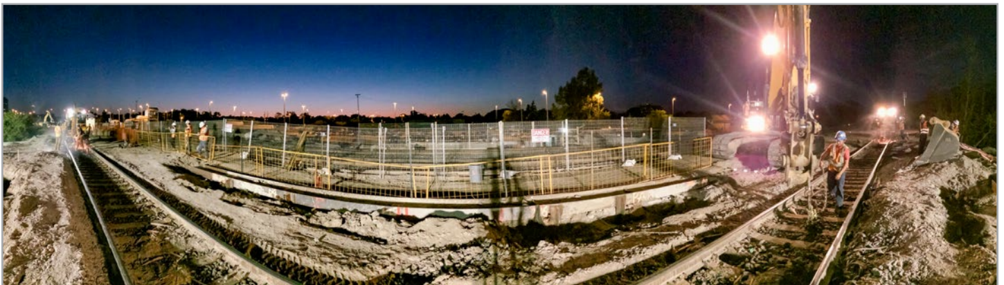
During a 53-hour weekend outage, PNR RailWorks track, signals & communications and GO Transit Maintenance crews helped with the installation of pedestrian tunnels near the GO Transit Guildwood Station west of Toronto.
