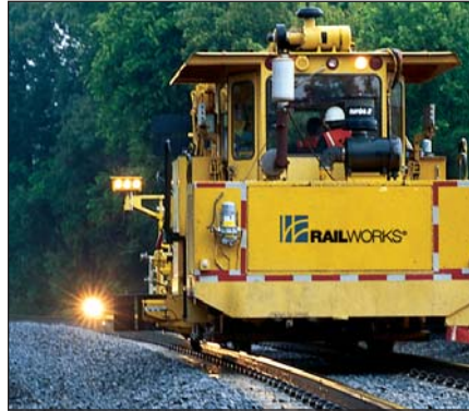
Railworks recommends using a tamper to resurface track every three to five years.
