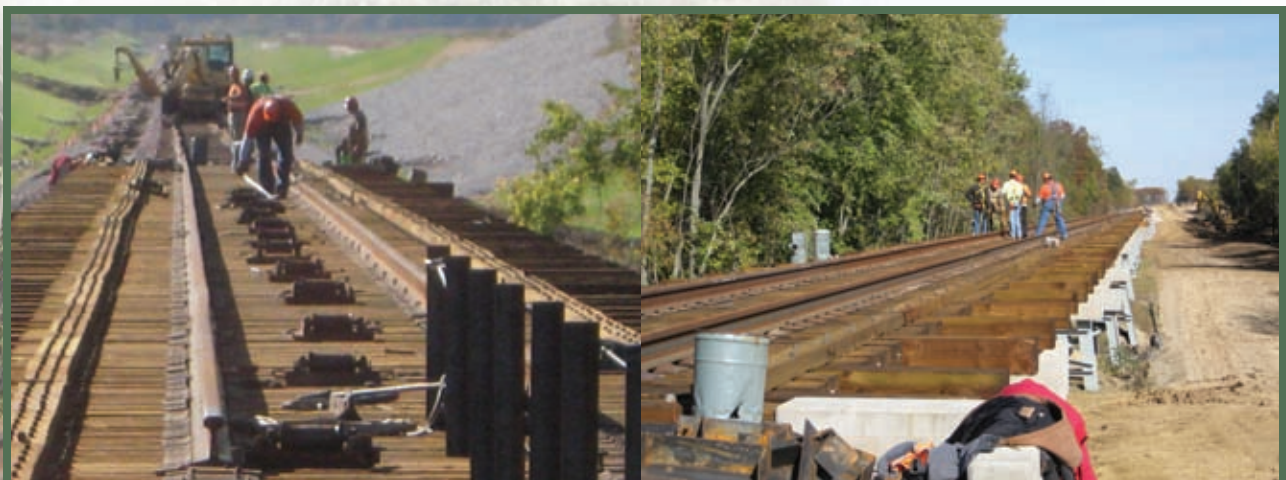
As of press time, RailWorks Track Systems Inc. was nearing completion on the first of a three-phase rail, bridge and earthwork project for Prairie State Energy Campus. RailWorks is performing the trackwork, grade crossing and signal construction work, furnishing all track materials, and managing the subcontractors performing the earthwork and bridge construction.
